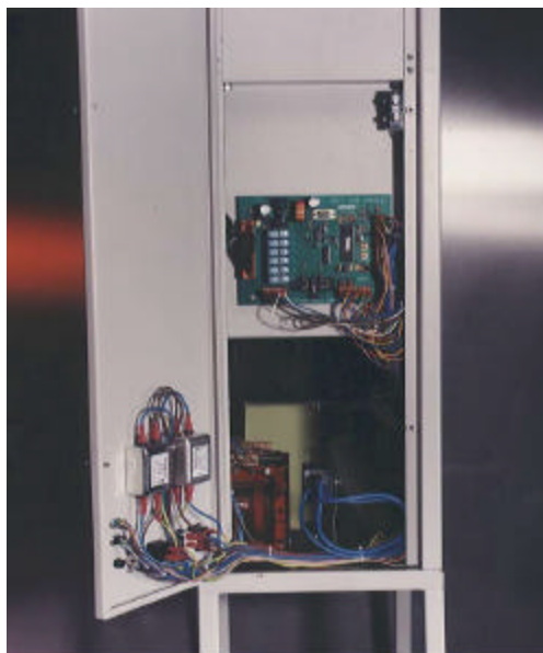
Rear of unit with door open showing the position of the controller camera and transformer.
